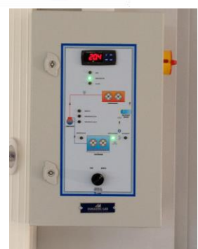
Control panel in cooler
